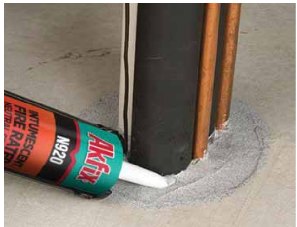
Hvac Penetration Cable-Pipe Sealing
