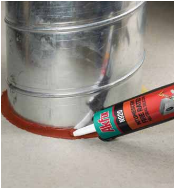
Fire Barrier Around Exterior Duct
