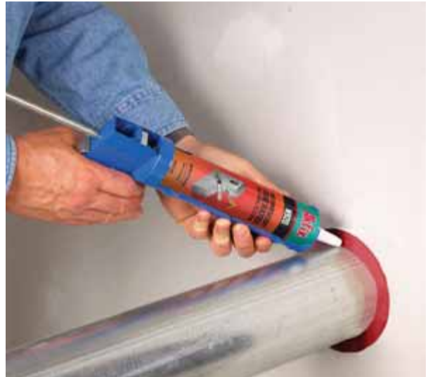
Combustible Pipe Sealing
