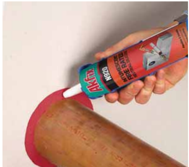
Combustible Pipe Sealing
